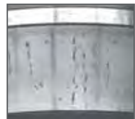
Rust and Corrosion
